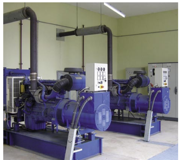
Two 250 kVA diesel generator sets for stand-by power supply at Akwa Ibom, Nigeria
