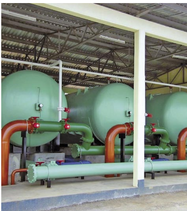
Horizontal pressure filters for iron removal incl. pipe work at Akwa Ibom, Nigeria
