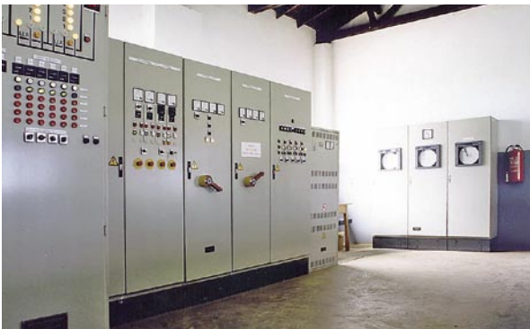
415 V motor control centre, control panel and flow meter panel in Kampala, Uganda
