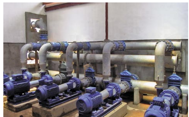
High Lift Pumping Station at Crossriver, Nigeria
